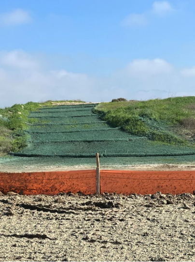
Photo 18 (pictured right) Haul Rd. about 0.25 miles east of Fairview Rd. Hydroseed, wattle and silt fence for erosion and sediment control BMPs.
