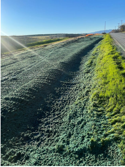
Photo 17 (pictured left) Fairview Rd near Basin B. Hydroseed and silt fence for erosion and sediment control BMPs. Improvements to existing natural drainage adjacent to Fairview.
