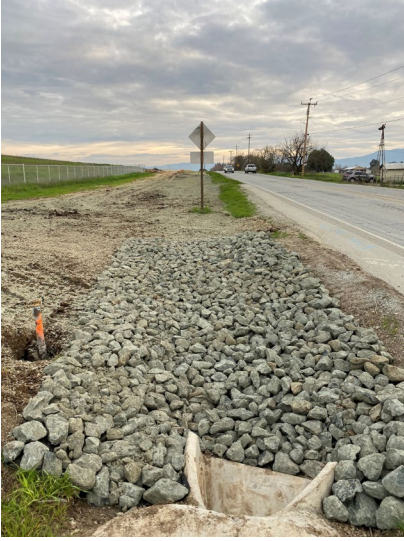
Photo 17b (pictured right) Fairview Rd near Basin B. Hydroseed and silt fence for erosion and sediment control BMPs. 4x8 rock apron on geo textile fabric at culvert. Improvements to existing natural drainage adjacent to Fairview.
