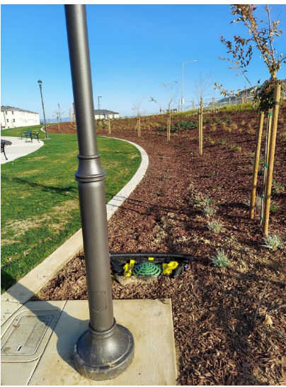
Photo 1 (pictured left) Community Park. Grass, landscaping and fabric filter installed below atrium grate for erosion and sediment control BMPs. Bark for ground cover.
