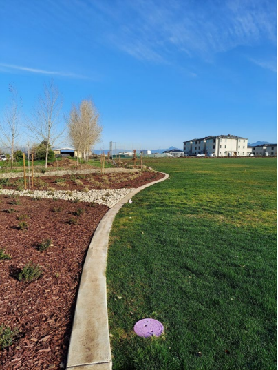
Photo 3 (pictured left) Community Park boundary, Cal Fire to the left. Grass, landscaping and bark for ground cover, 2x4 rock placed in swale with fabric filters below atrium grates.
