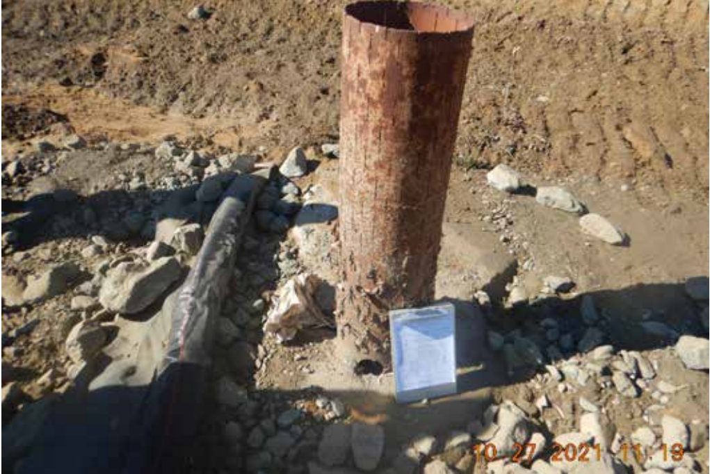
Photo 13. Standpipe in linear basin seen in Photo 12. 4.5 ft tall, 16-inch diameter reused slotted steel well casing. Note one of four 3-inch diameter holes cut at base of casing. Clipboard is 14x9 inches.
