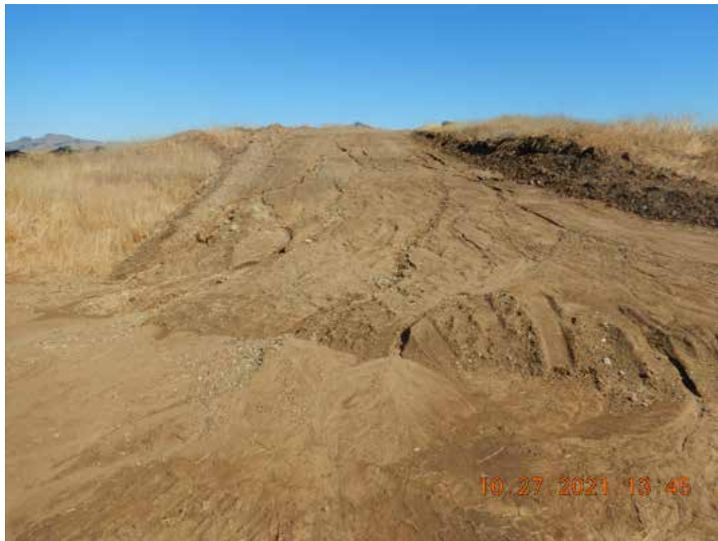
Photo 18. Haul road for demolished buildings about 0.25 miles east of Fairview Rd. Note lack of erosion and sediment control BMPs, deep rills and sediment fans. Central Coast Water Board staff inspection photo.
