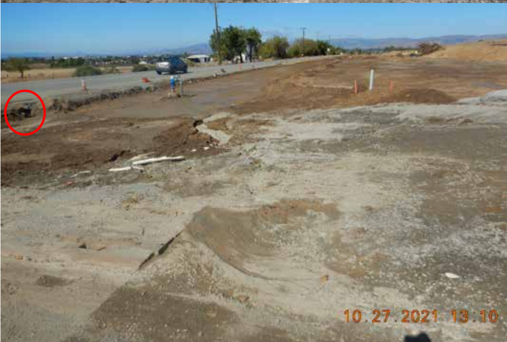
Photo 16. Hillcrest Rd. at Fairview Rd., showing sediment accumulation and sedimentary flow structures. Note lack of erosion and sediment control BMPs. Red circle is location of pipe under Fairview Rd. Central Coast Water Board staff inspection photo.
