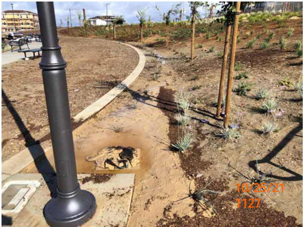
Photo 1. Community park area near toe of slope from Santana Ranch Rd. (right); note siltation and mulch, clogged drop inlet, and lack of erosion and sediment control BMPs.
