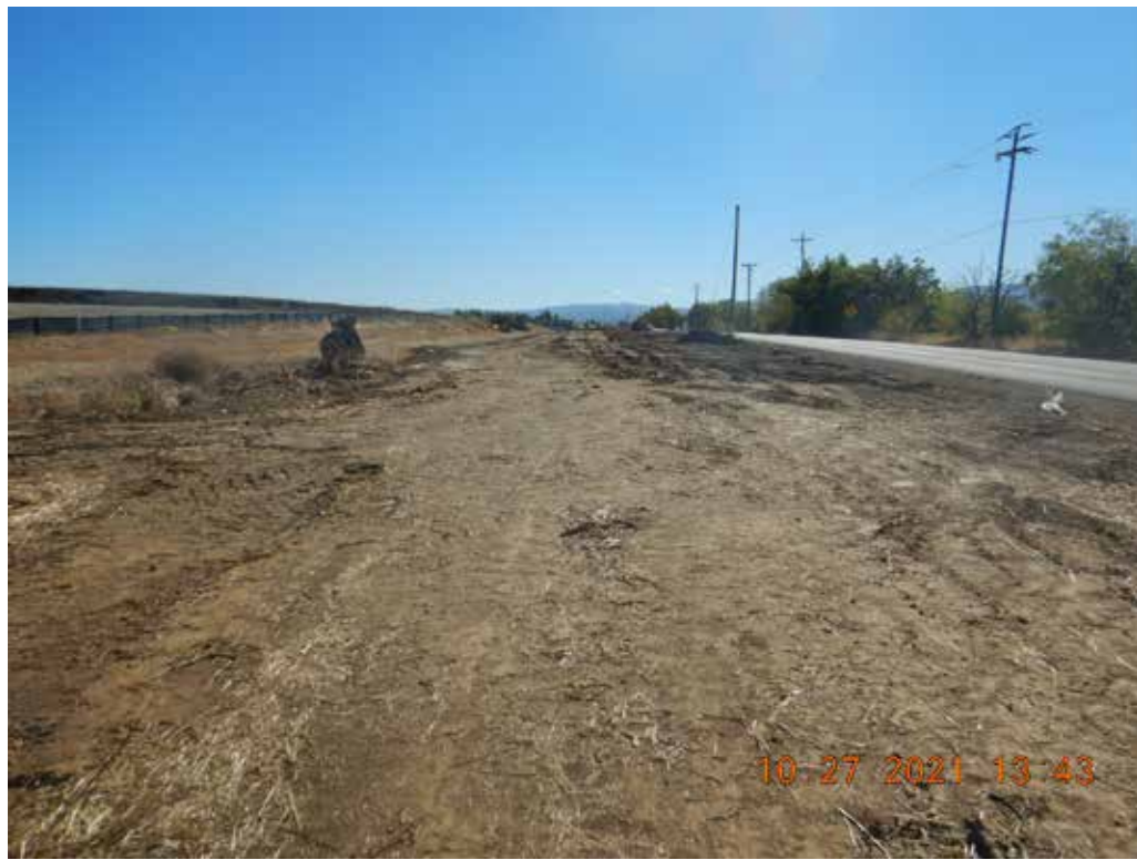
Photo 17. Cleared land east of Fairview Rd. Cleared land stretches from Cal Fire station (approx.) to Basin B, approximately 2,200 feet by about 80 feet wide. Note lack of erosion and sediment control BMPs. Central Coast Water Board staff inspection photo.
