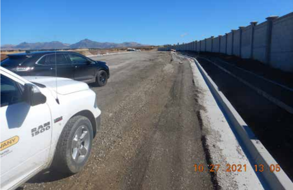
Photo 14. East extension of Hillcrest Rd. from Fairview Rd., showing evidence of concentrated flow in aggregate base along gutter. Note lack of erosion and sediment control BMPs. Central Coast Water Board staff inspection photo.
