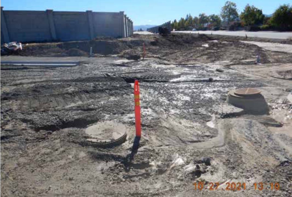
Photo 15. Hillcrest Rd. at Fairview Rd., showing sediment accumulation and sedimentary flow structures. Note lack of erosion and sediment control BMPs. Central Coast Water Board staff inspection photo.
