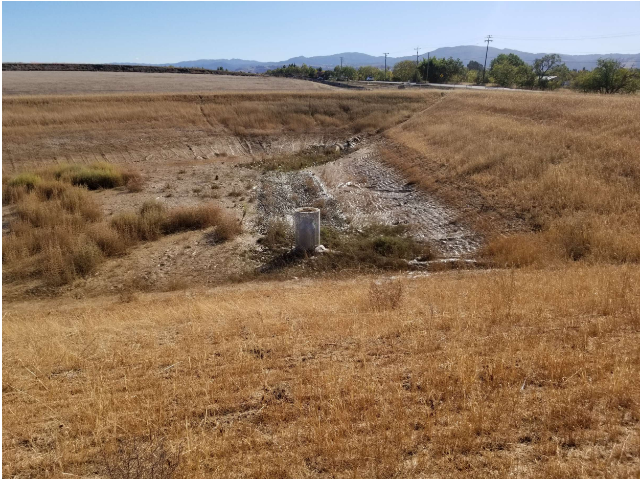
Figure 11. Basin B-35.jpg – Basin B outlet Riser
