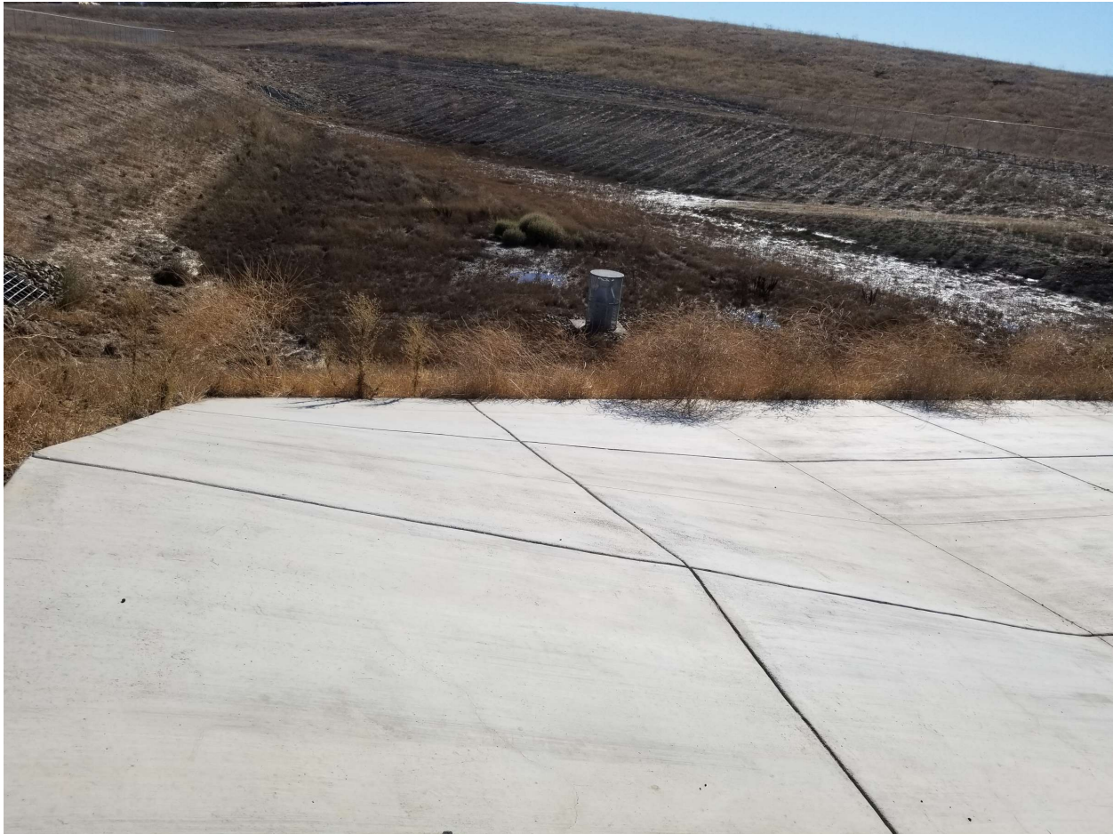
Figure 9. Basin A-19.jpg – High water mark
