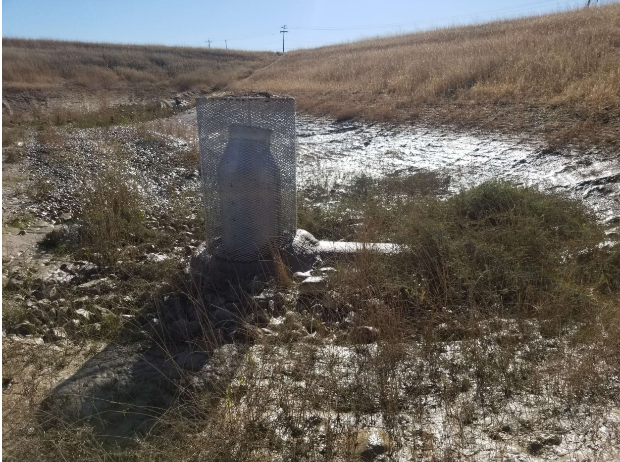
Figure 12. Basin B-38.jpg – Basin B outlet Riser with high water mark
